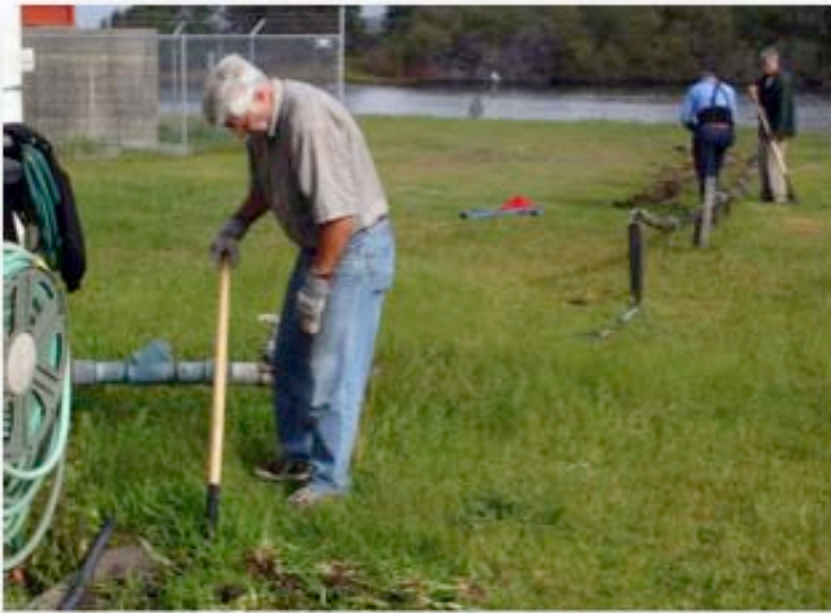
Jim Bradt, Larry Drees, and Al Norman dig a trench to bury our new sump pump line
