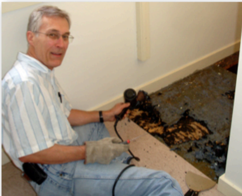
Walt Hayden tackles the slow and tedious job of removing the old floor from the upstairs bathroom
